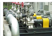
KTM Installed in parallel system
